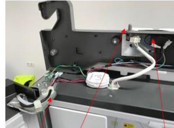
Water hose switch
