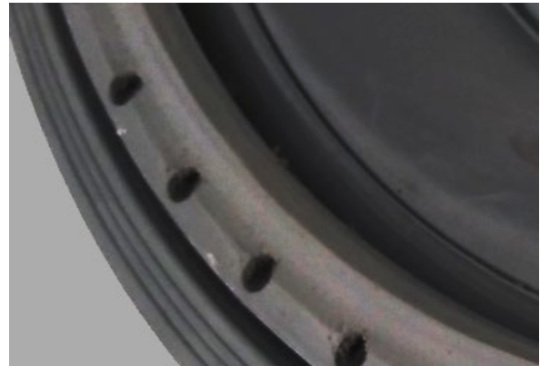
Rubber bellow with visible signs of erosion due to friction between the gasket and the drum's front flange
