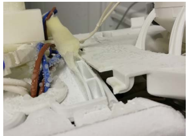
2. Fan unit is not in the right position.
