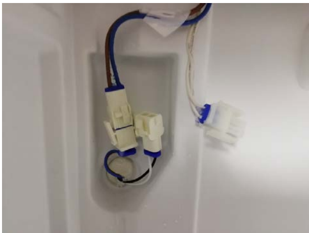
1. Fan is not connected
