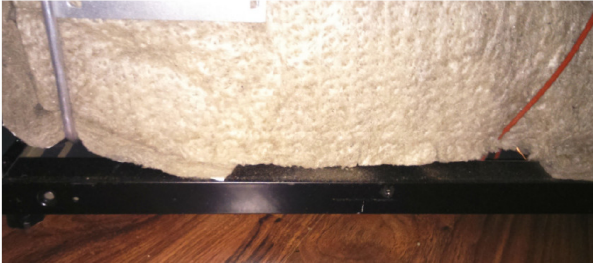
Insulation at rear is touching the base support
