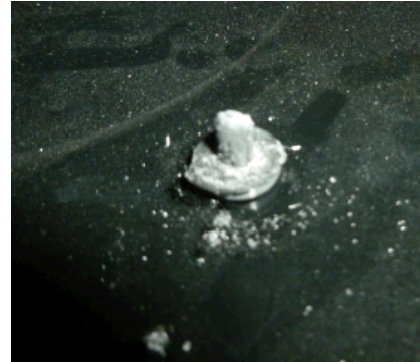
Deteriorated old type of rubber feet
