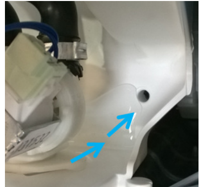
Photo3. Leakage through hole in gutter.
