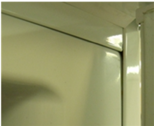
Curved inner liner corner. Possible cause of excessive icing.
