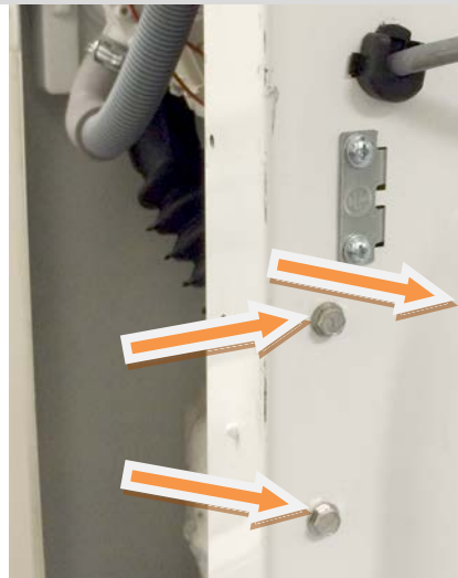
Unfasten screws securing UIMC board to the cabinet.
